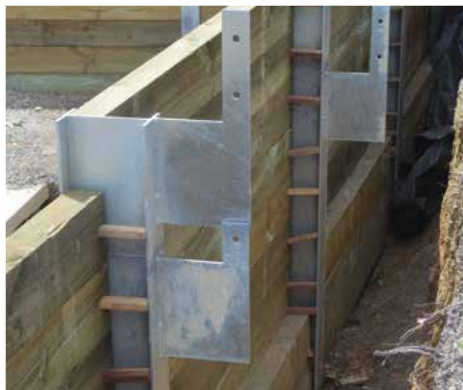
Offset fencing brackets were used to properly locate the fence on the boundary
